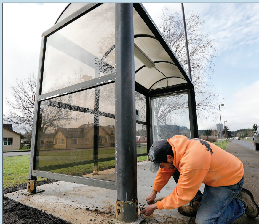
CG Contractors LLC employee Todd Fitzgerald secures a bus shelter to a concrete pad while installing it in Tribal housing on Thursday, Feb. 22.
