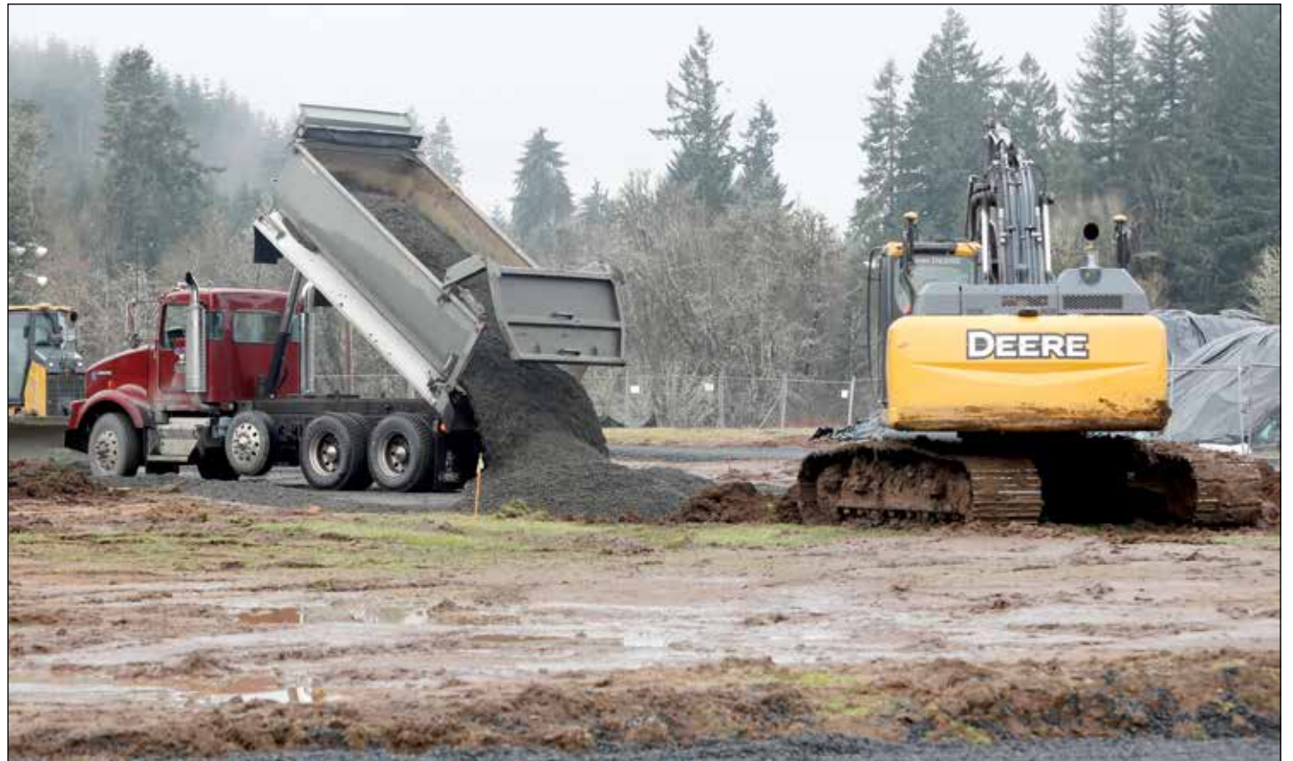
A truckload of gravel is dumped during construction of the child development center on the Tribal campus on Thursday, Jan. 25. Construction on the 26,000-square-foot building, located next to the Tribal gym, began in December 2023 and is expected to take a year.
