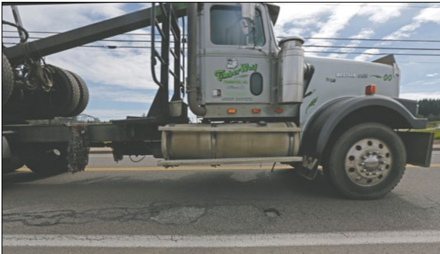
A truck drives over a repaired pothole on Grand Ronde Road on Monday, April 22. Heavy truck traffic is taking a toll on the road, which was rebuilt a little more than a decade ago.
