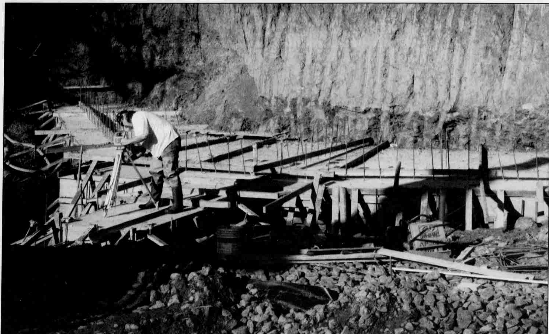
Tribal member Tim George, with Round Valley Construction, takes some measurements for the next phase of the job.
