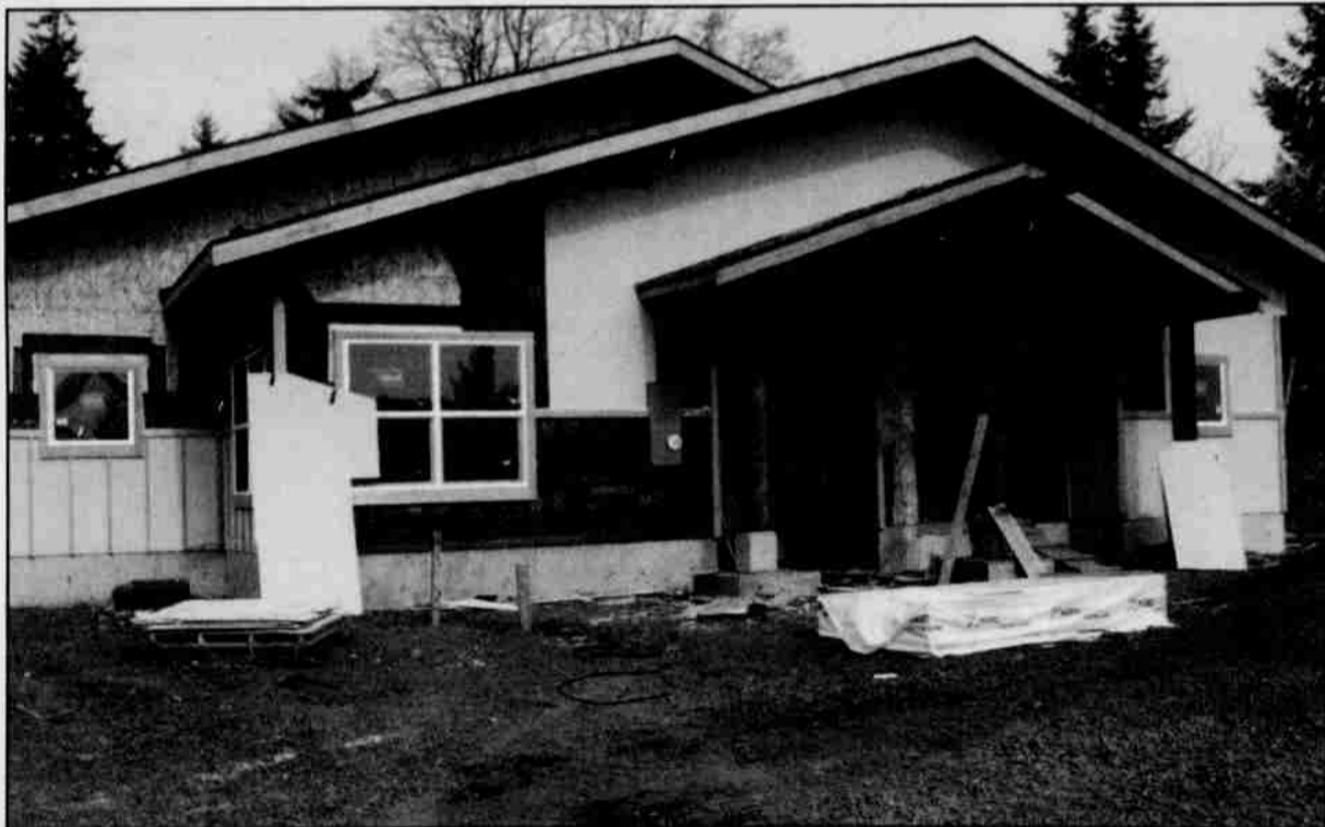
Homeplace — Early Spring weather has been a blessing for making progress on the Elder Foster Care Facilities and has made it possible for the project to be well ahead of schedule. One of three initial buildings is seen here in a photo taken on Thursday, April 7.
