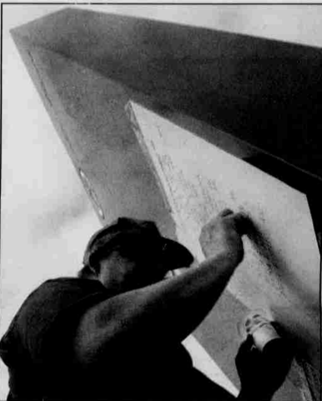
New Names Added —Kelly Breeding of Oregon Memorials works on one of the 20-foot black granite obelisks. Granite is the third hardest substance known, after diamonds and sapphires.
