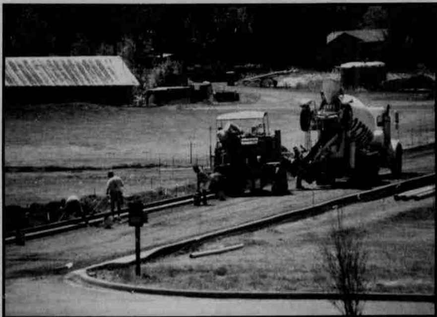
Access Improves — Construction crews pour curbs for a new access road being built this summer on the Tribal campus near the pow-wow grounds.
