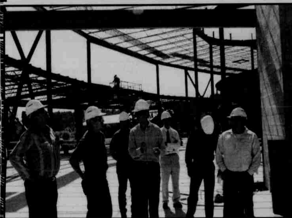
A foundation for self-sufficiency: Bruce Thomas shows off the casino construction site to Tribal Council.
