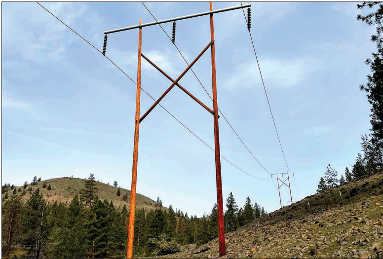
The current Bethel-Round Butte transmission lines run 98 miles between the reservation and the Willamette Valley. The lines are supported by wooden power poles, while the new lines, with much greater capacity and efficiency, will be supported by metal poles.
