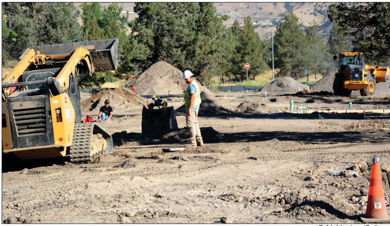
Infrastructure and foundation work last week at the Permanent Supportive Housing construction site.
