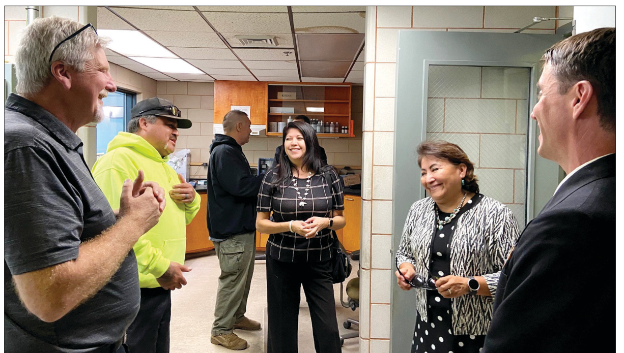
Utilities general manager Chico Holliday (second from left), IHS director Roselyn Tso (second from right) and the leadership team tour the Dry Creek water treatment facility, slated for improvements.
