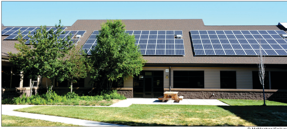
The central courtyard area of the Warm Springs Academy, with its rooftop solar panel component.
