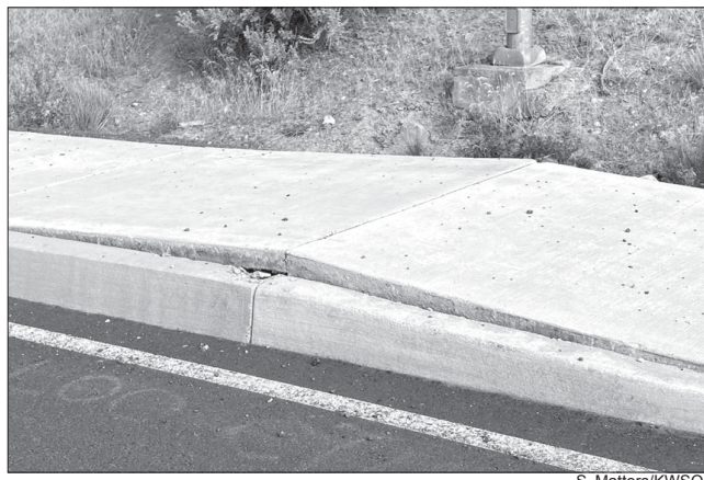
Sidewalk in Warm Springs pushed up by the heat.
