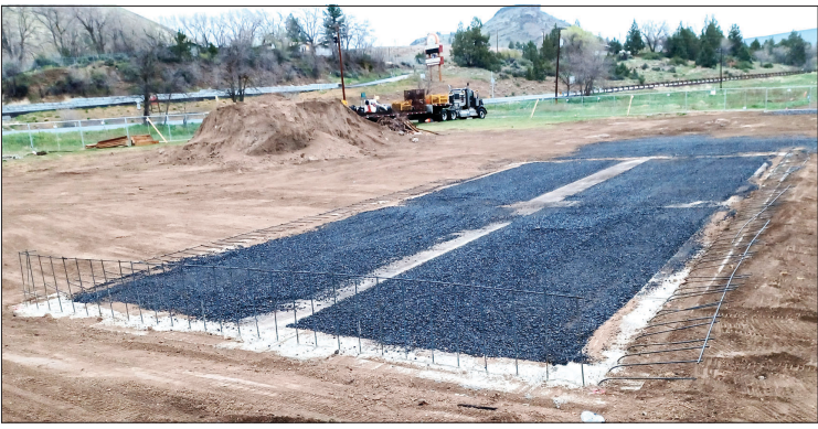
This was the foundation made for the Commissary Business Incubator. The Warm Springs Community Action Team and the tribes had Kirby Nagelhout Construction create the foundation pad over the past several weeks.
