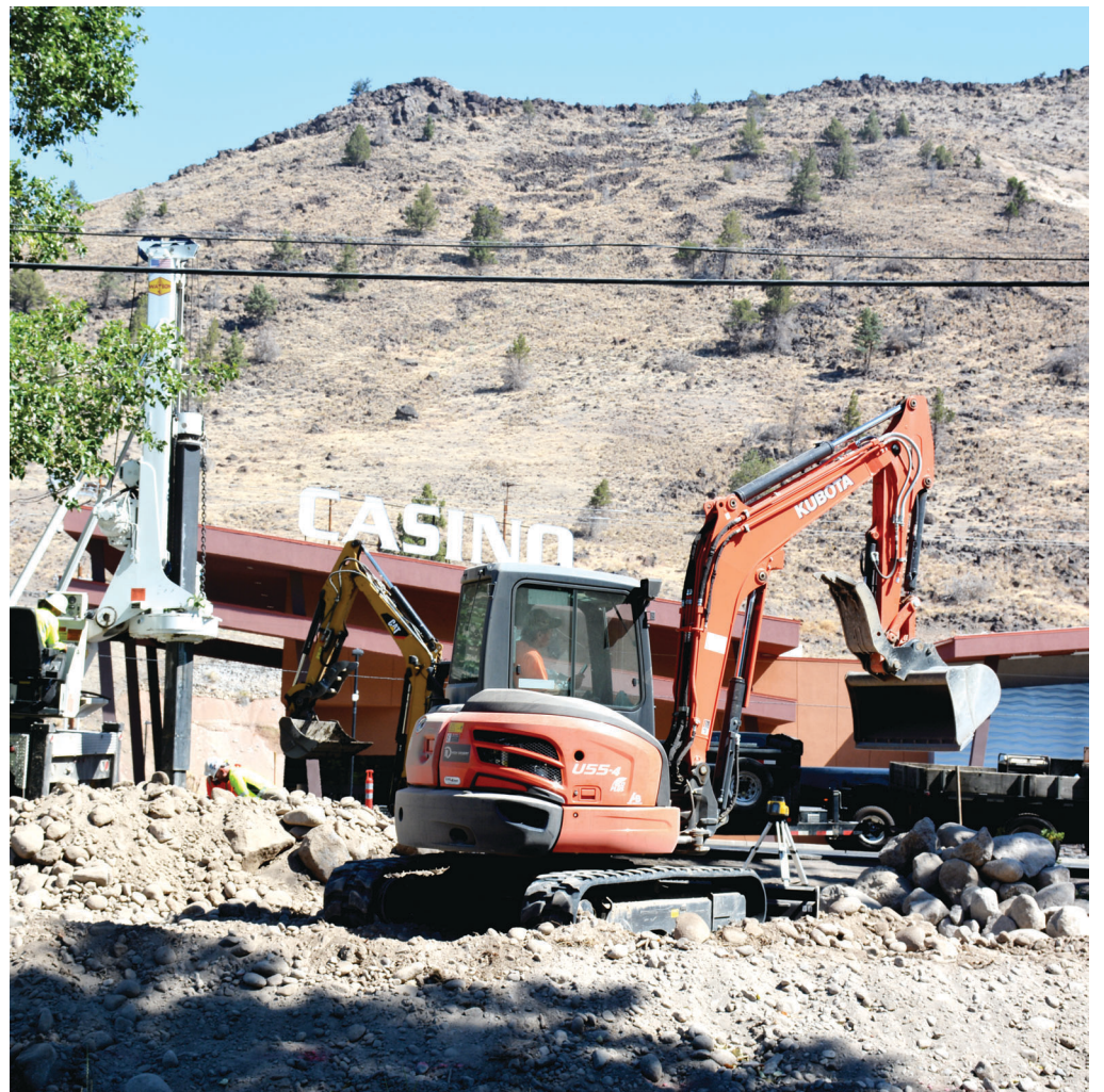
View of the Highway 26 construction project from the area of the Museum at Warm Springs, looking toward Indian Head Casino.
