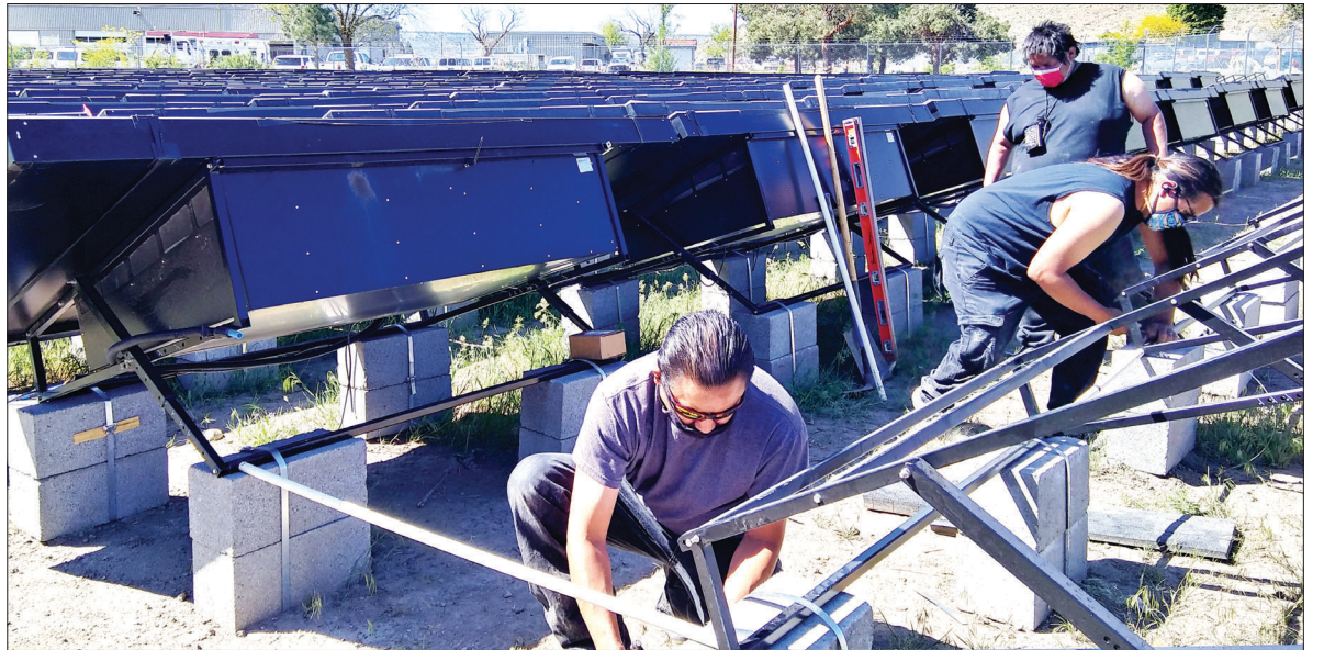
Warm Springs Construction crew—Jeremy KillsFirst, Warner Williams Jr. and Warner Williams Sr.—installing frames for a new set of Source solar-water panels.
