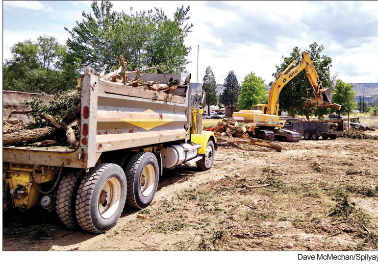
The Warm Springs Construction crew removed the trees from the future home of the Small Business Incubator building.
