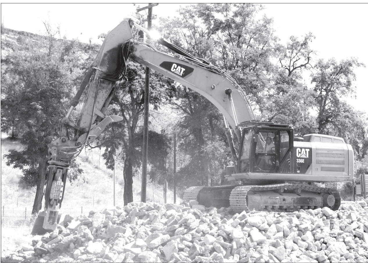
Work continues this week on phase 2 of the downtown demolition and removal project. The BIA-fund project is removing a number of unused and condemned buildings on campus and elsewhere in Warm Springs. Here, the foundation concrete of the old Spilyay building is being broken up before being hauled away.
