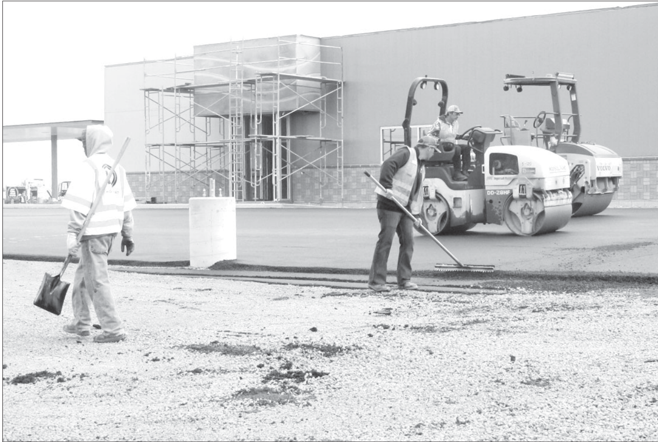
The construction crew puts down the asphalt paving at the Plateau Travel Plaza.
