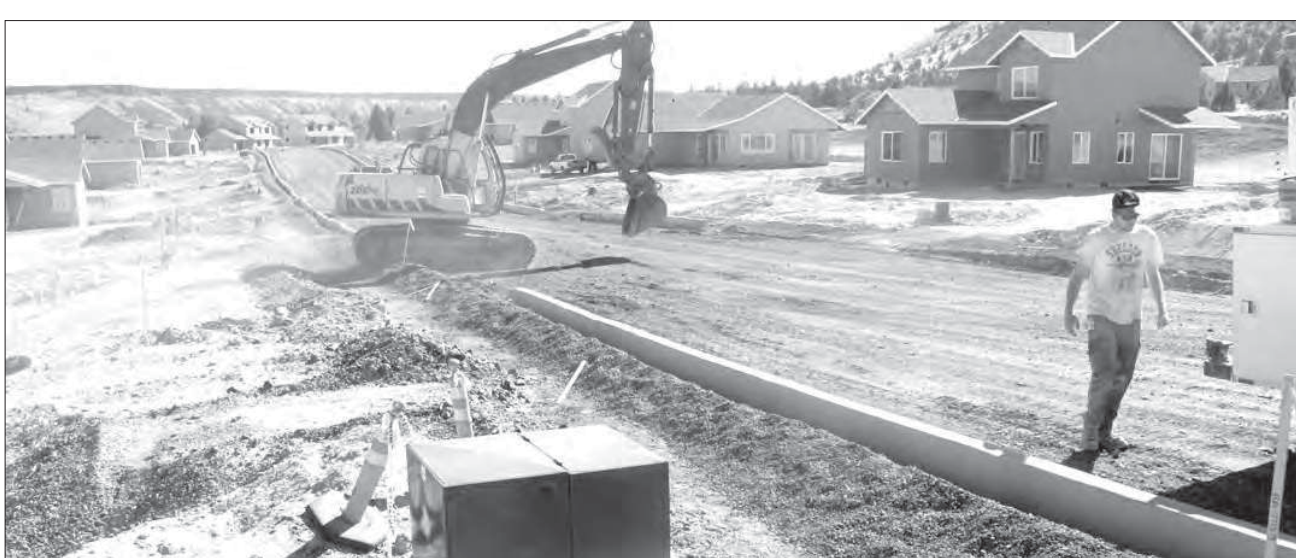
Curb, sidewalk, road and other construction work continues at the Greeley Heights subdivision, the 35-unit project of the Warm Springs Housing Authority.
