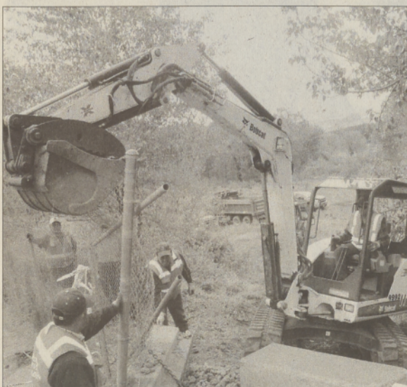
BIA Roads workers repair the fence on the Hollywood Boulevard bridge over Shitike Creek.
