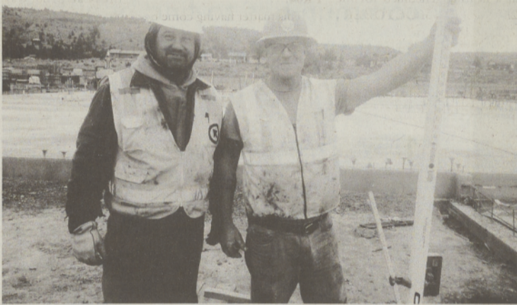
Clint Bruisedhead of Warm Springs and Jim Smith of Redmond at work on the Warm Springs K-8 School.
