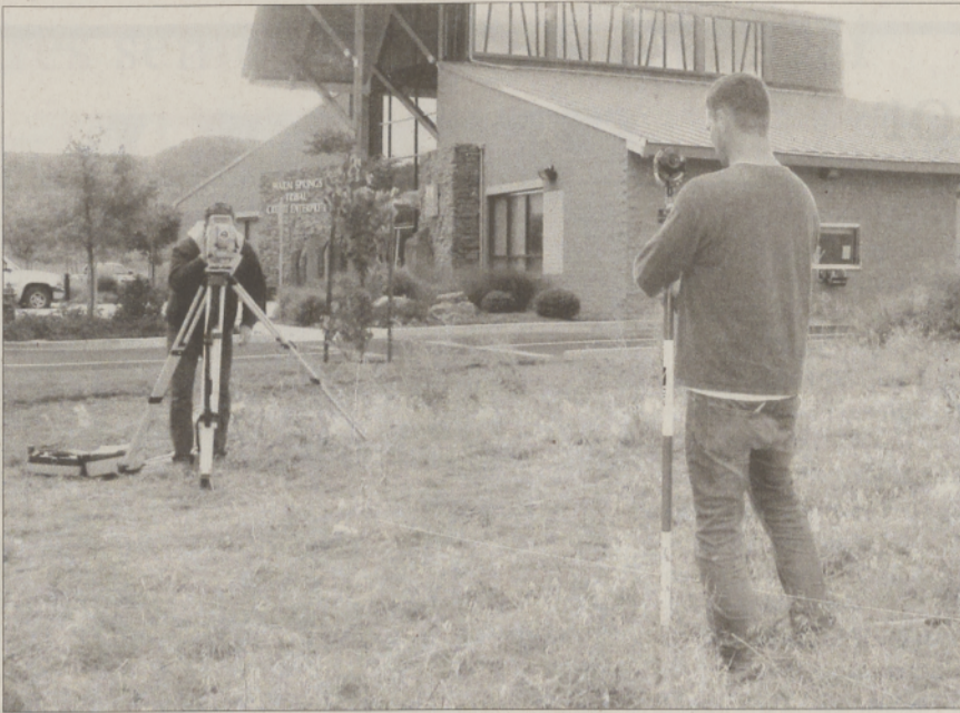
Surveyors with the company plot the ground for the solar cells by the Credit enterprise building.
