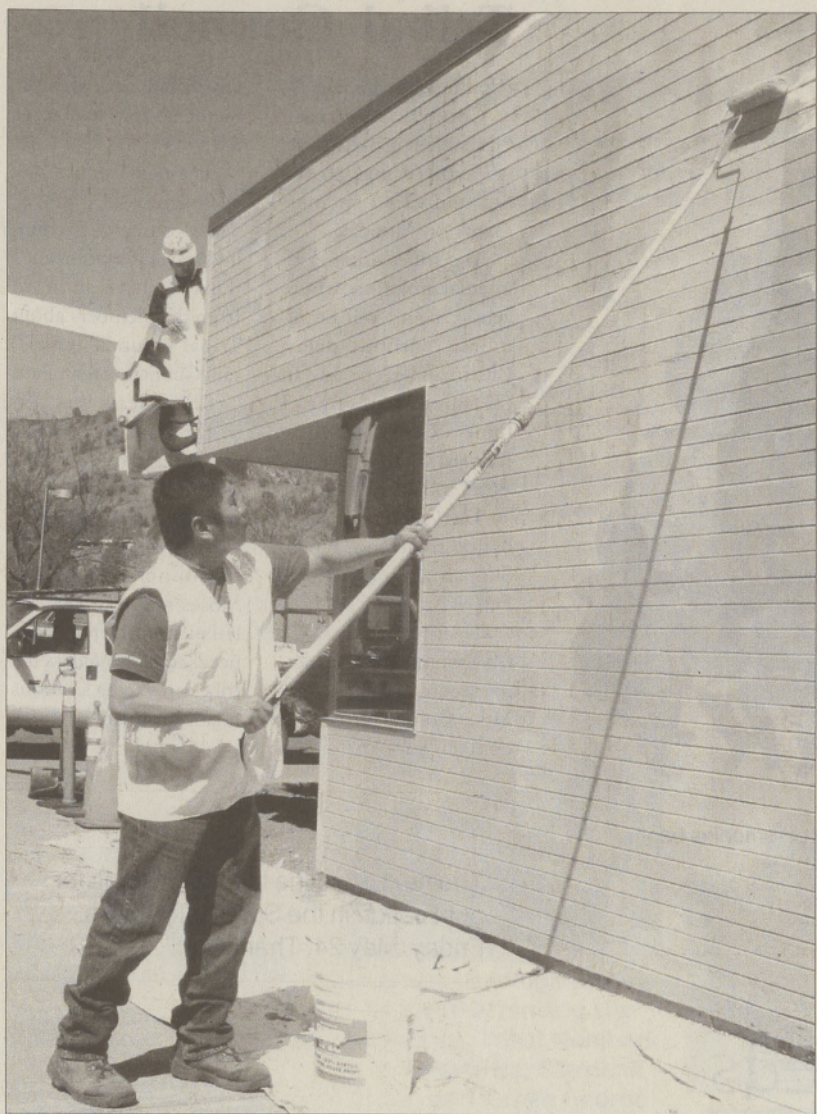
Utilities maintenance foreman Alvis Smith III and Jerrod Allen (in lift) paint the tribal administration building, in preparation for the Council swearing-in ceremony.
