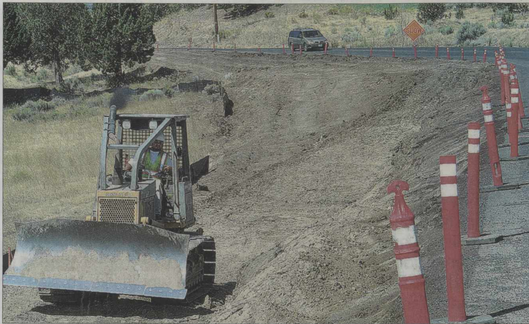
A construction team is working on a walking trail beside West Hills Drive. BIA Roads is funding the project, currently under construction.
