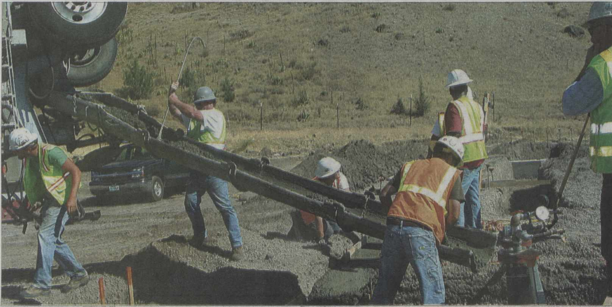
The construction crew poured the foundation of the building last week and earlier this week.
