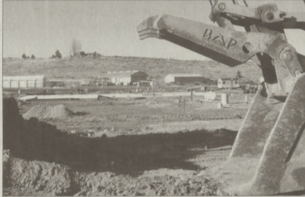
The tribal Construction crew is working at the Fire Management building site.
