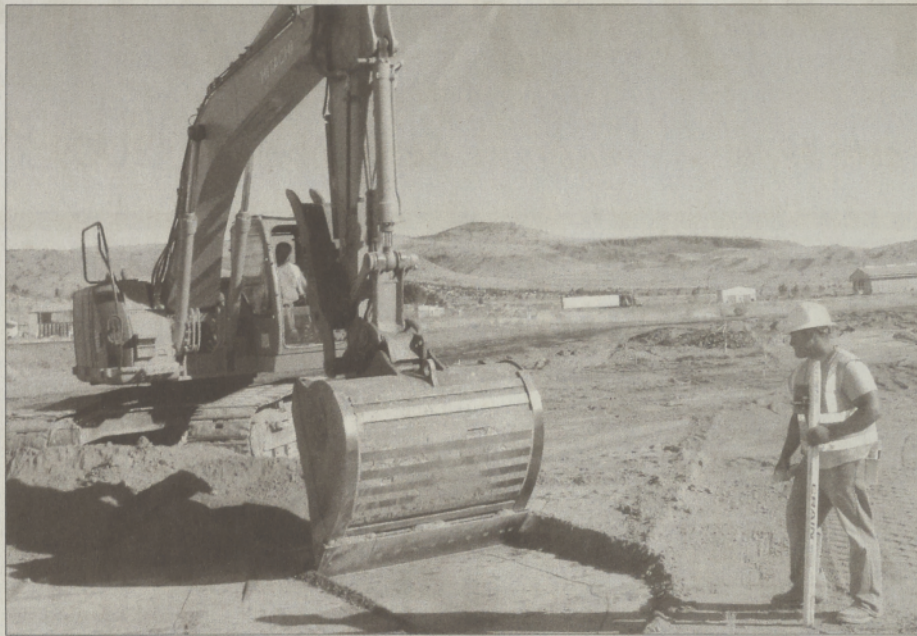
Kevin Hernandez and other Warm Springs Construction crew members are working on the Fire Management building.
