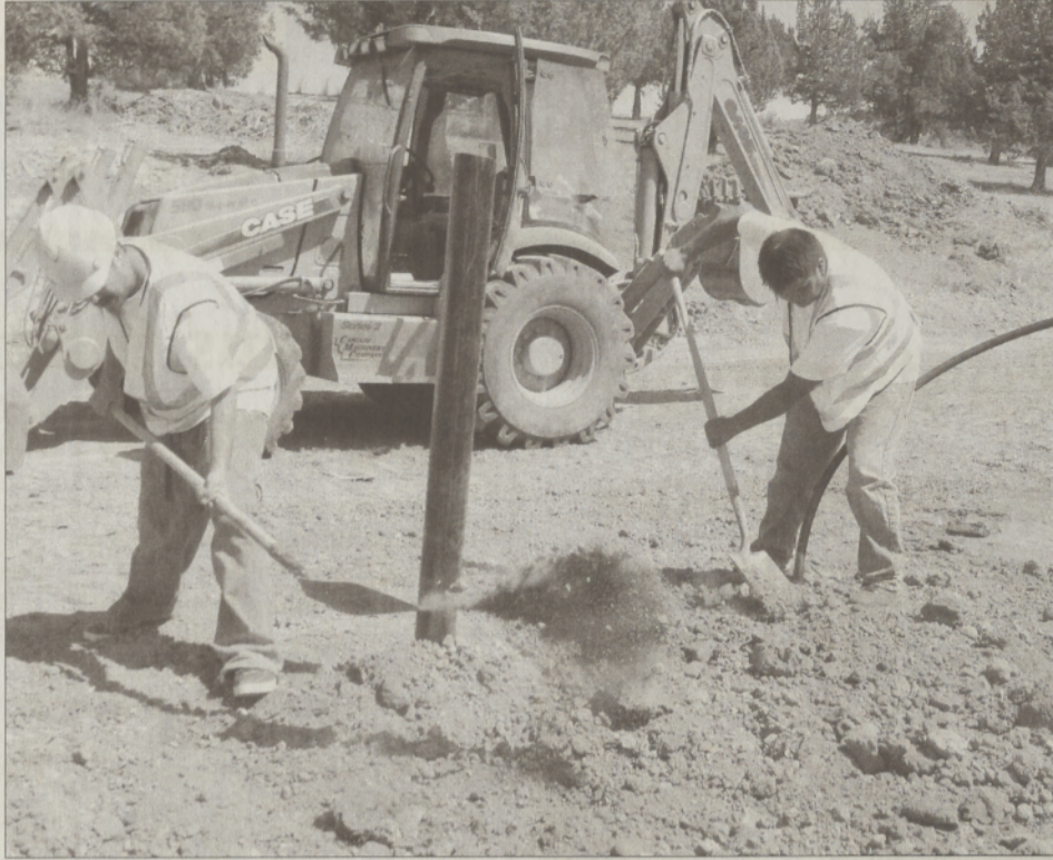
Housing construction workers Nathan Williams and Kanim Smith prepare the site for one of the new modular homes.
