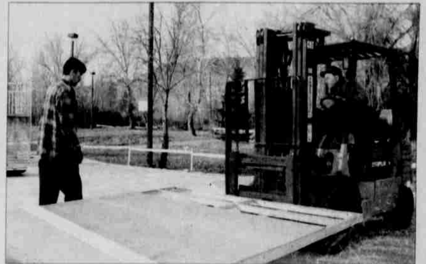
Workers from skate park developers Spohn Ranch Inc., of Calif., built the Warm Springs skate park earlier this week.
