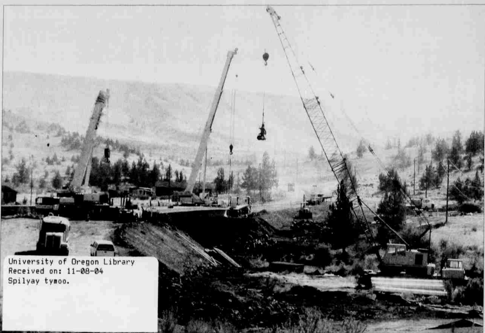
Construction crews place the large beams across the river at the new bridge by Kah-Nee-Ta.
