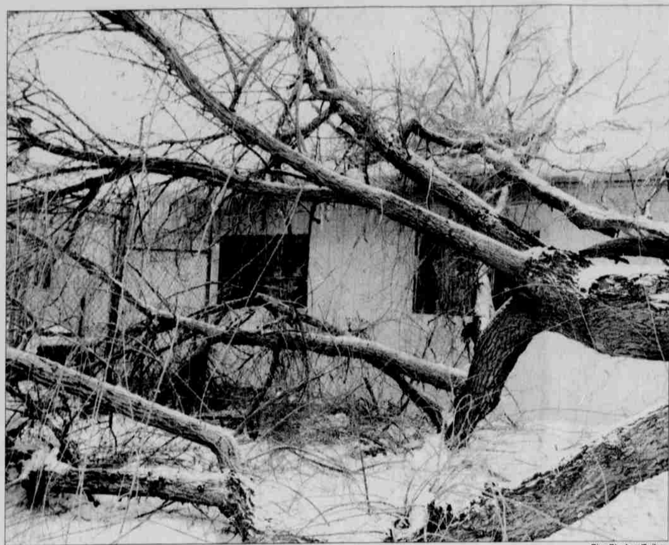
Bing Bingham/Spilyay During the recent snow storms, a tree fell on the Children's Protective Services building. No one was in the building at the time, and there was no structural damage, though there was possible damage to a heat pump.
