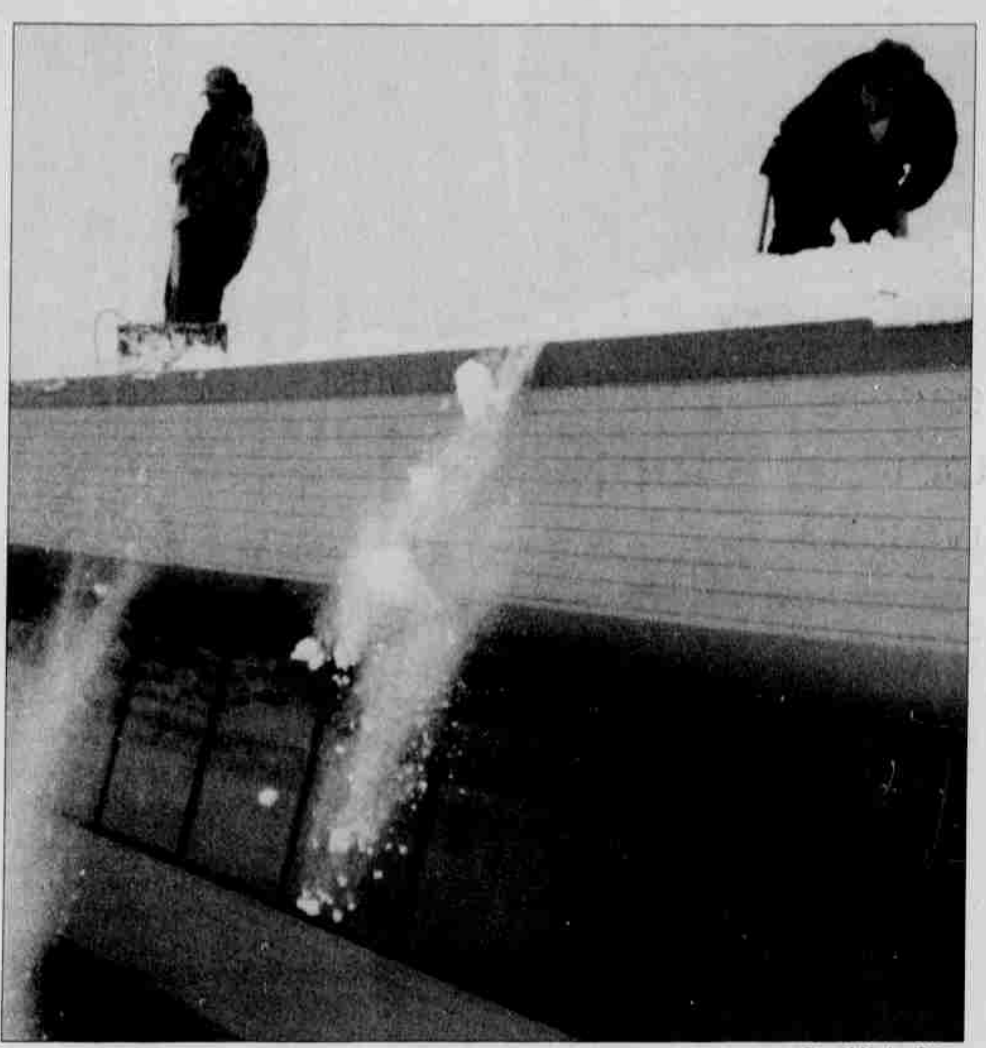
A maintenance crew clears snow that had accumulated on the roof of the administration building. Maintenance workers were kept busy for several days, clearing roads and pathways to tribal buildings.
