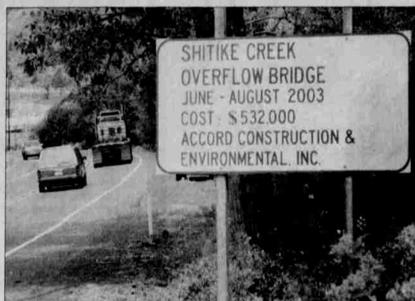
As the ODOT sign along the highway indicates, the overflow bridge project will take about three months, and will cost about $532,000.
