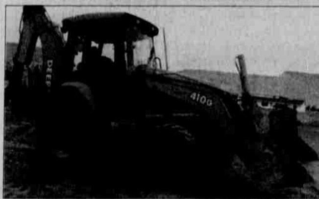
Crews with the Warm Springs Construction enterprise are working on the Bear Drive housing construction project, which will bring 25 new homes to Warm Springs. At top, Frank Reese buries a new water line that will serve the houses. The heavy machinery is being operated by Derrick Flowers.
