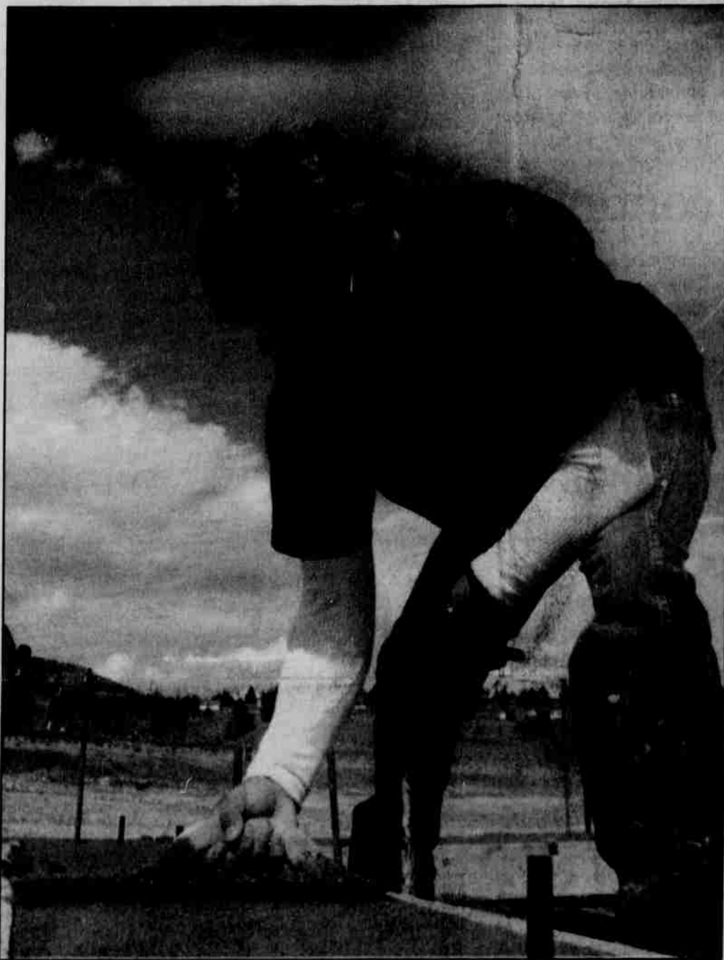
A construction crew with Workforce Development, including Ricky Smith (above), is working on three new homes in the Sunnyside area. New homes are needed to meet demand.
