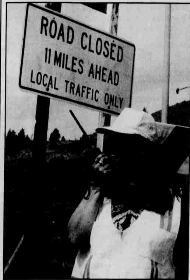
Beverly Arthur is working for the Oregon Department of Transportation, helping direct traffic to the detour around the Mill Creek Bridge project.
