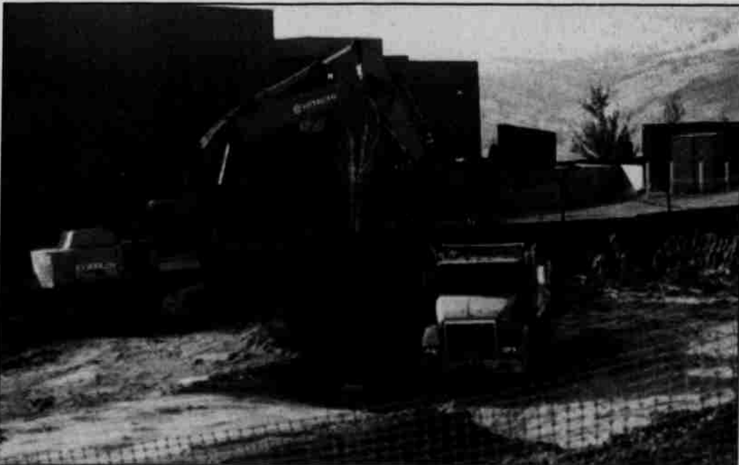
Kah-Nee-Ta Resort is undergoing a $5 million renovation project. As part of the project, 107 rooms will be remodeled. The work is scheduled for completion in March 2002.
