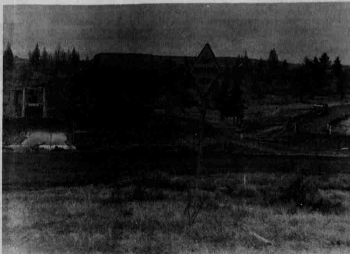
Road construction in the Lower Dry Creek area started early last month and will continue as soon as the weather permits
