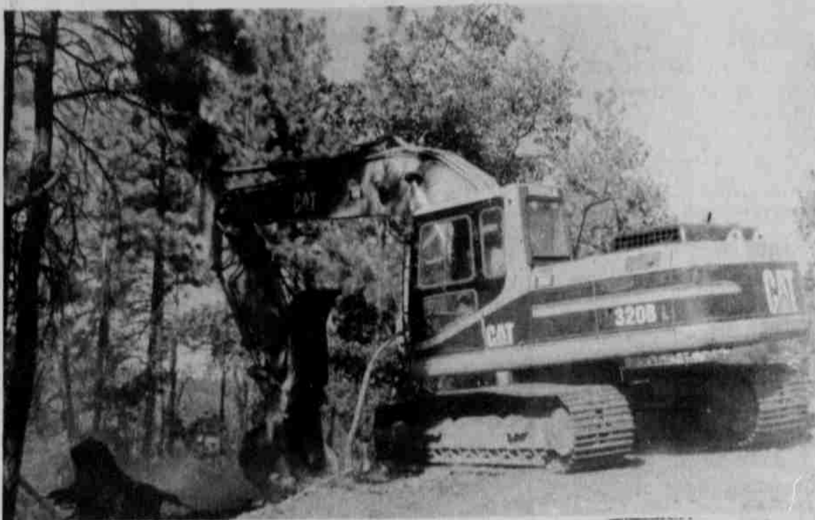
Using heavy equipment and a hand crew, restoration work is done by putting dozer lines back to bed
