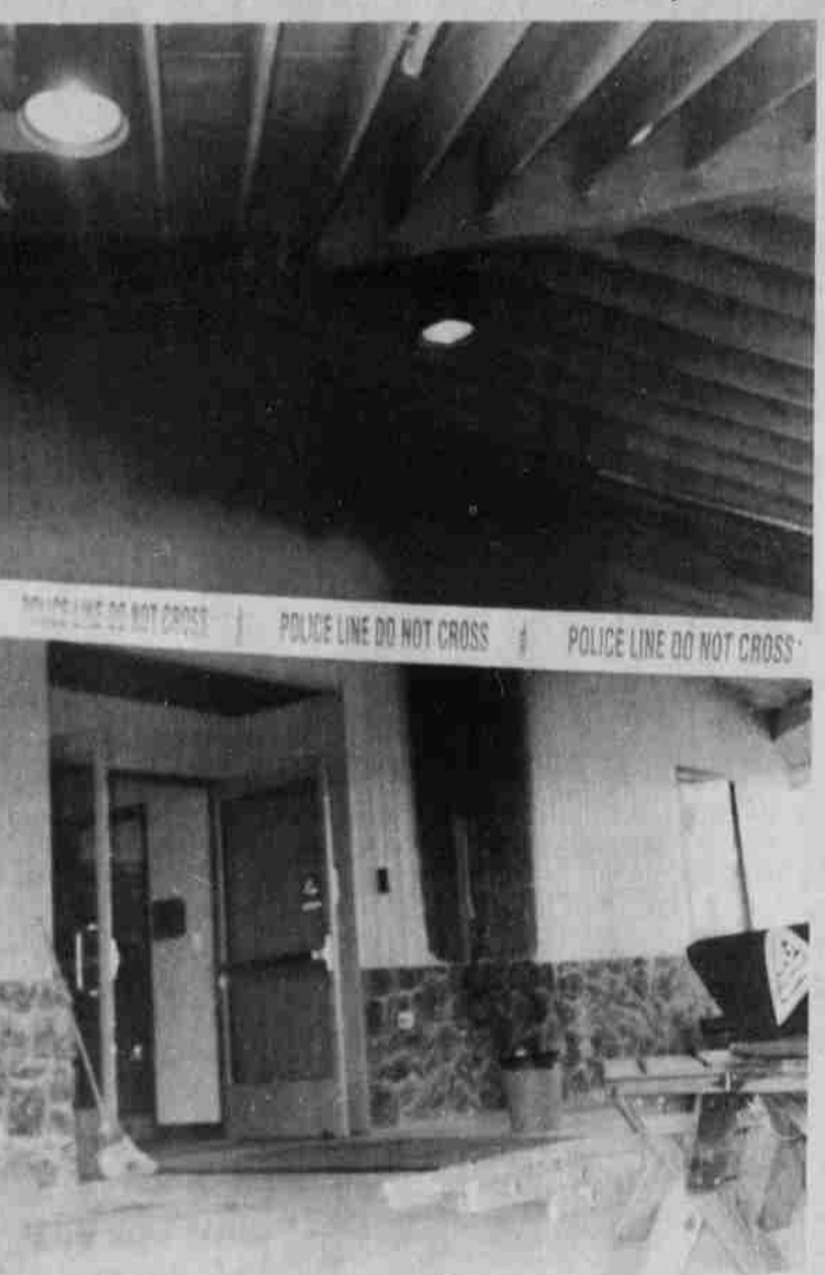
Fire began from the trash can outside the eastside of the building
