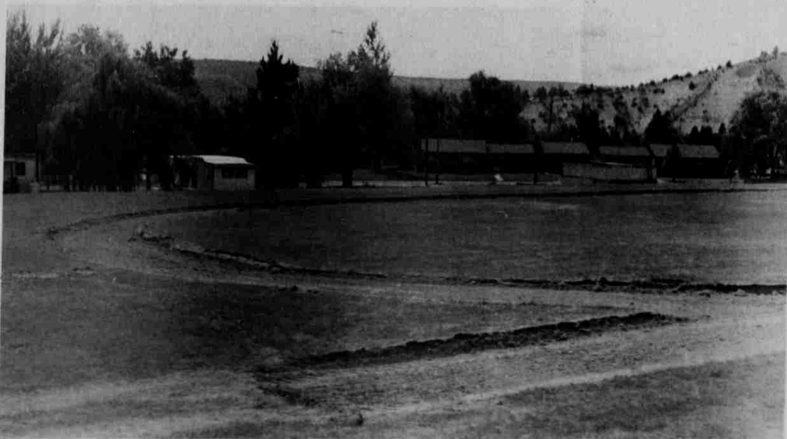
Warm Springs Elementary began construction of new track near the upper playground.
