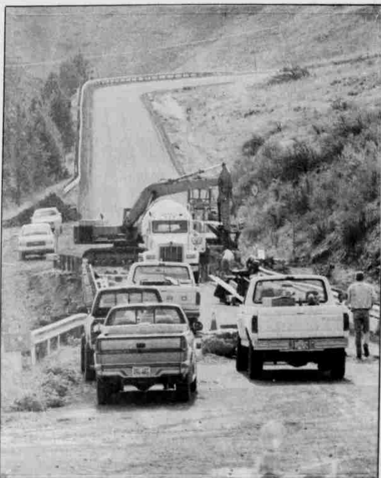
On Friday April 12, a contract to rebuild the Warm Springs Bridge on Route 3 was awarded to the tribal Construction department. Prior to this time, much effort has been expended designing repair plans and securing funding for the flood repair work. Work begun on Monday April 15. Preliminary schedules predict this work to be completed in approximately 30 days. The foundation and concrete pours should be done by April 26. The tribal construction department and BIA Roads department is working closely with the Natural Resource department to minimize the impacts to the environment. Use of the Wolf Point detour will continue until completion of this project. The road user's patience when using the detour after the flood damage to the bridge has been appreciated.
