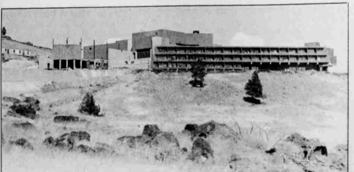
Construction work on the permanent Indian Head Gaming facility is moving along now that inclement weather seems to be a thing of the past. Gaming officials have stated the permanent facility will be open in October.
