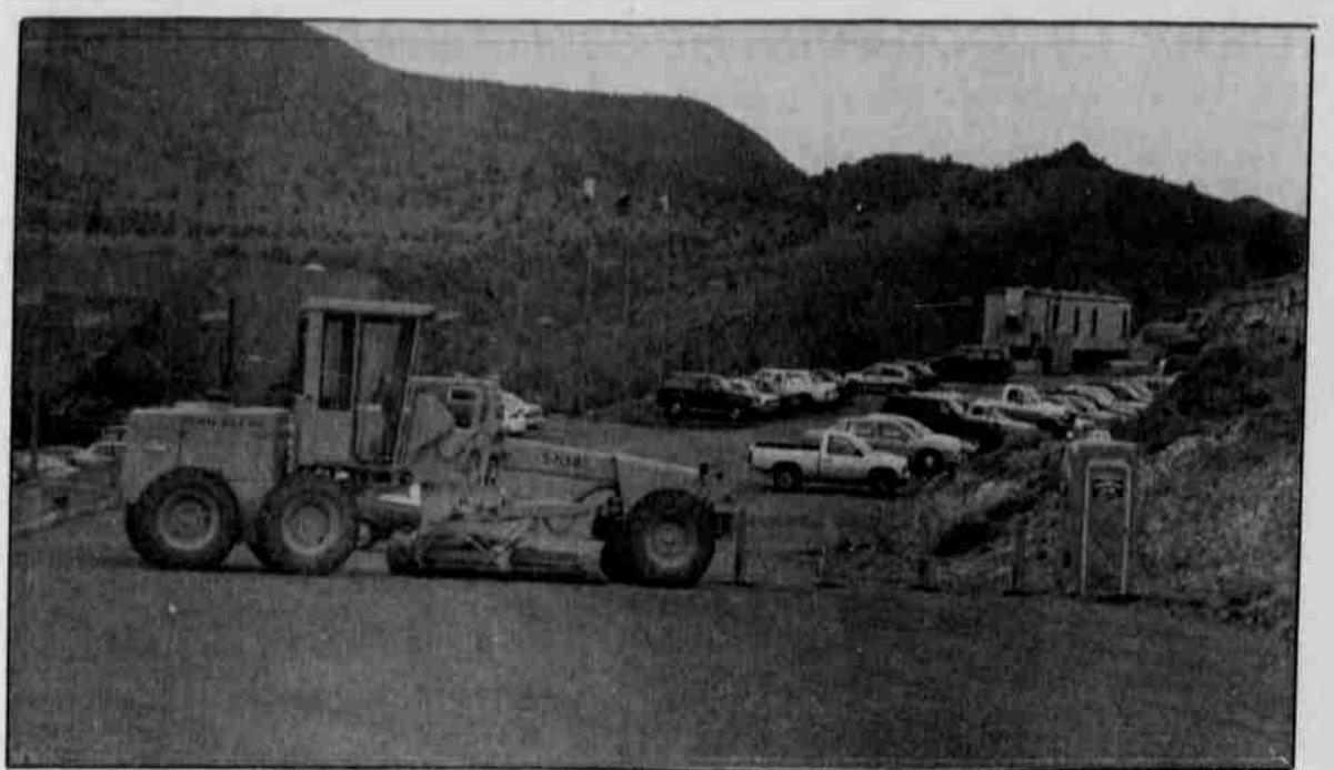
Preliminary work began about two weeks ago near Kah-Nee-Ta Lodge to make room for the gaming facility. Work on the temporary spot, in the current Wasco and Paiute Rooms, will begin April 11 with the opening set for May 1. The temporary facility will have nearly 150 machines. The permanent facility is expected to open late this summer. Frontier Construction is the primary contractor for the facility.
