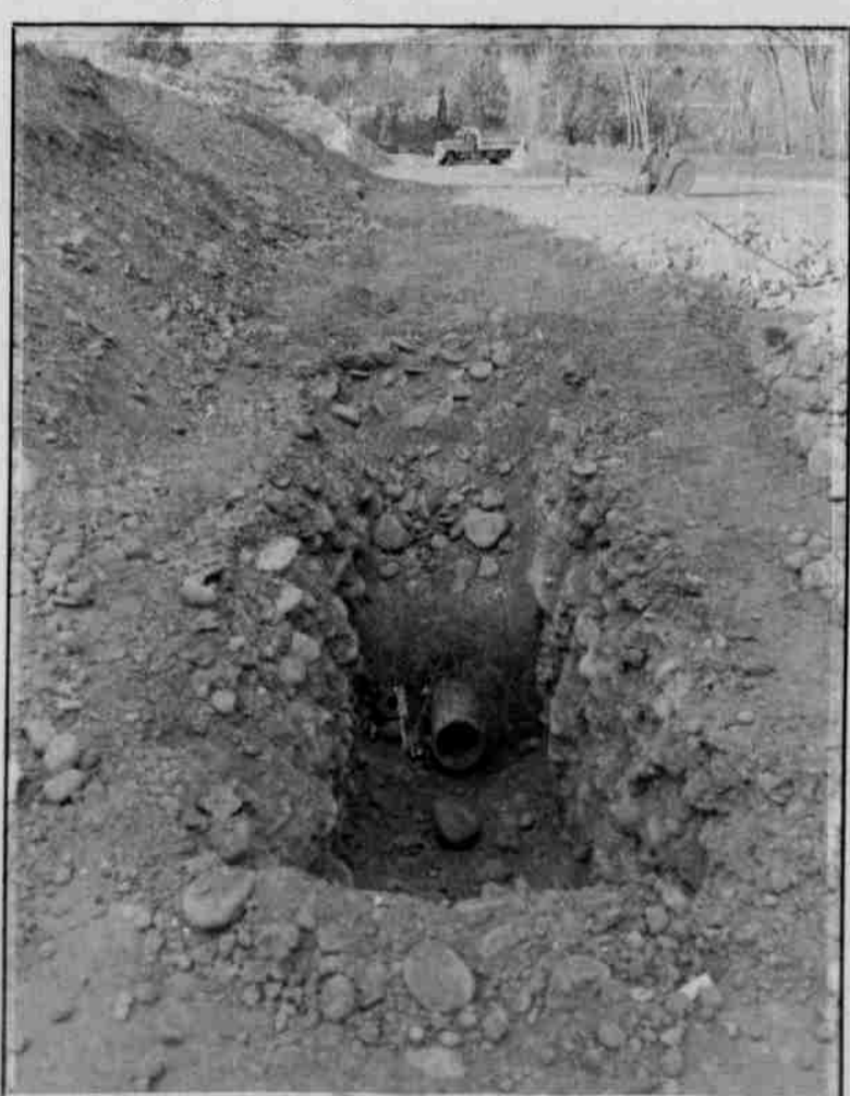
A $960,000 dollar Sewer Project is under construction along highway 26 which was made possible by a fifty percent loan, fifty percent grant from the state of Oregon Lottery Monies. Completion is expected to be the end of February 1995.
