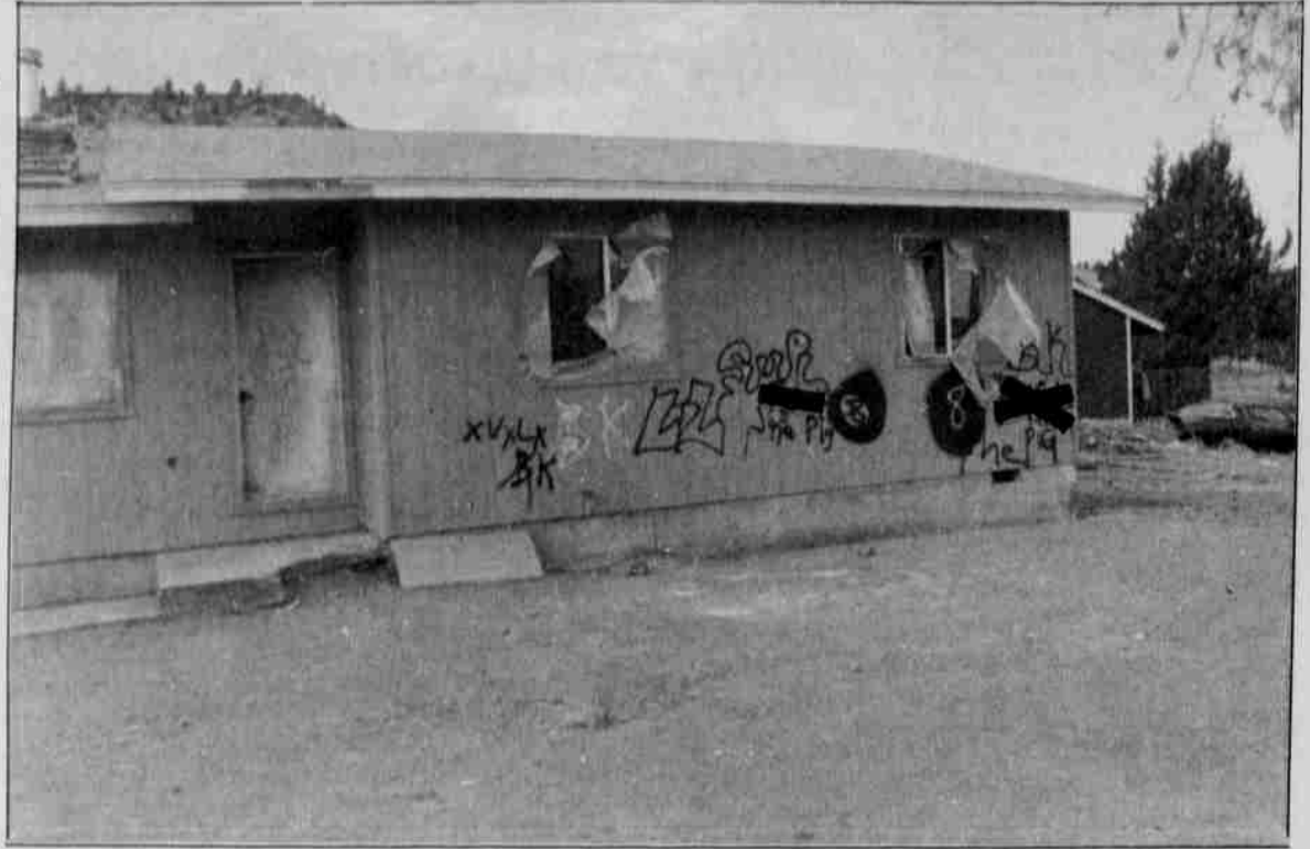
The former Kalama house at 1791 Tao-shuh Ave. was severely damaged by a fire, March 11, 1994. Renovation began July of 94 by Housing general contractors. The house, 80 percent completed, was marked by graffiti for the second time this month.
