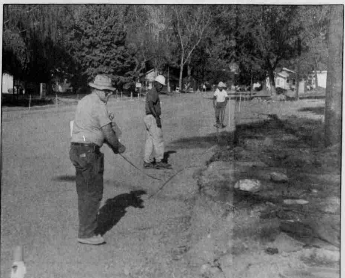
Dick Souers, and crew prepare to put in cement curbs throughout the campus area.
