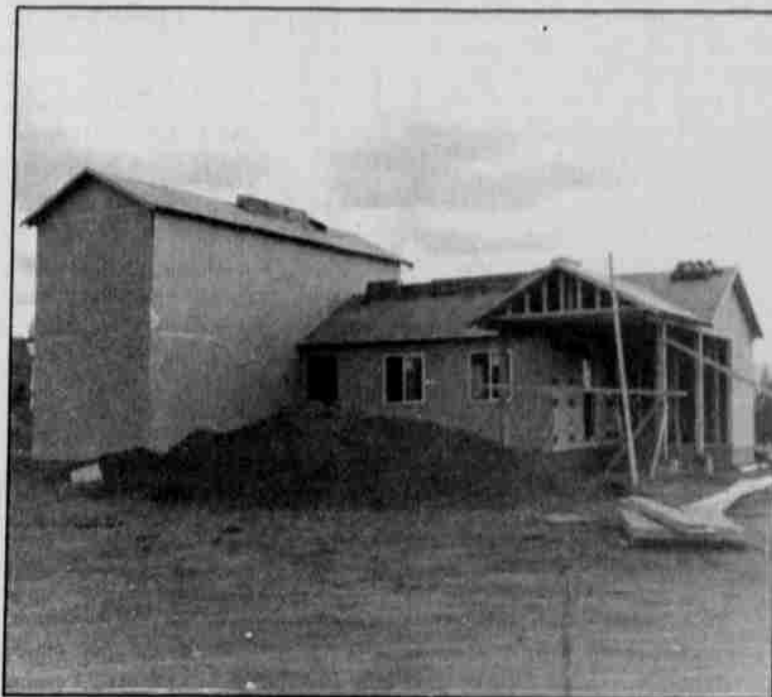
Photo by Saphronia Katchia Fifteen Mutual Help Homes are near completion. The first few homes will be ready for move in, in a couple of weeks. This one in particular belongs to John Jr. and Saphronia Katchia, which was taken in June.
