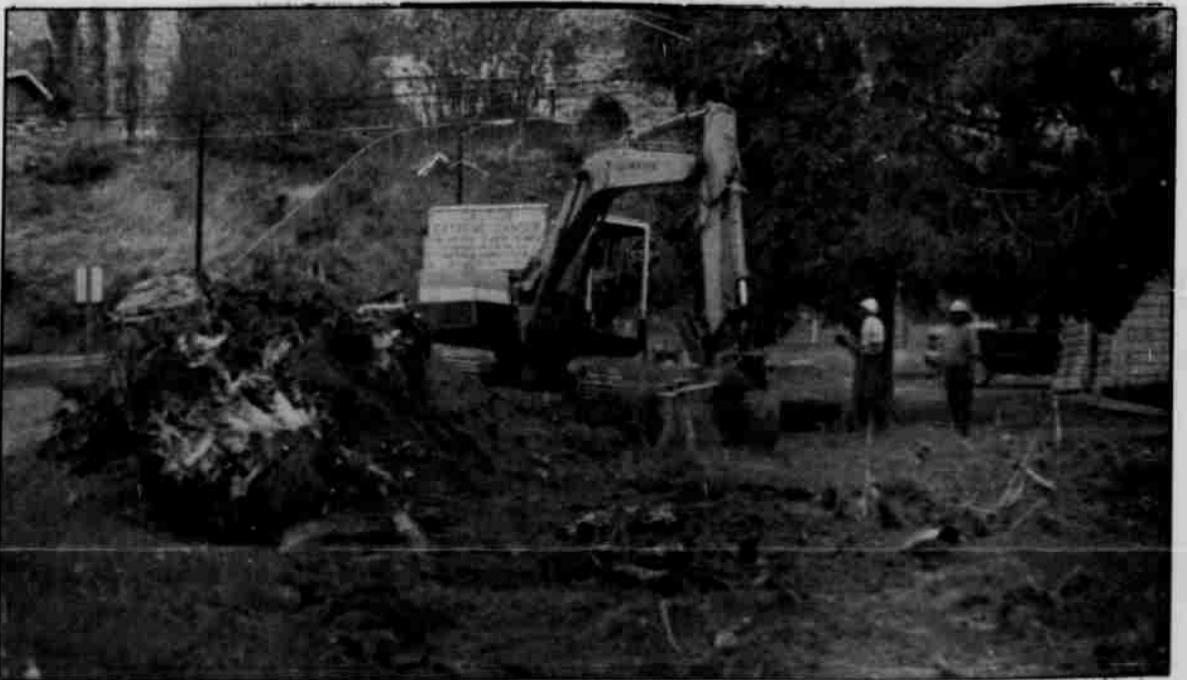
Construction crews removed the poplar tree trunks adjacent to Paiute Street last week. Work continues on the renovation of Warm Springs and Paiute streets.
